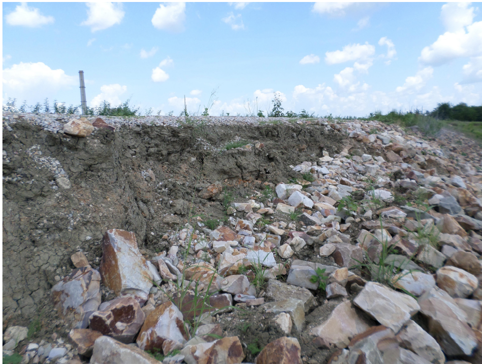
No. 2 - Scarp of the Slide Near the Crest of the Embankment
