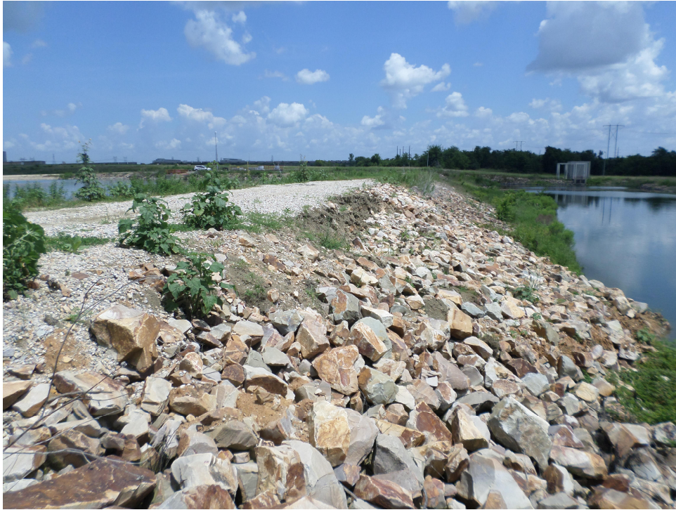
No.1 - Slide on Downslope of Embankment
