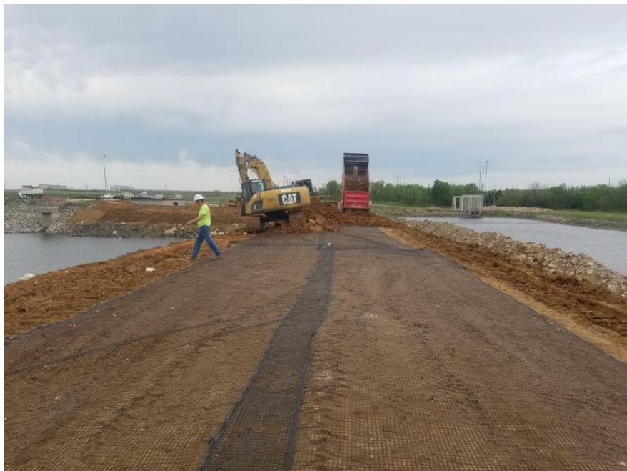
FIGURE 12: ADDITIONAL LAYERS OF GEOGRID AND FILL ARE PLACED TO BRING EMBANKMENT UP TO FINAL GRADE
