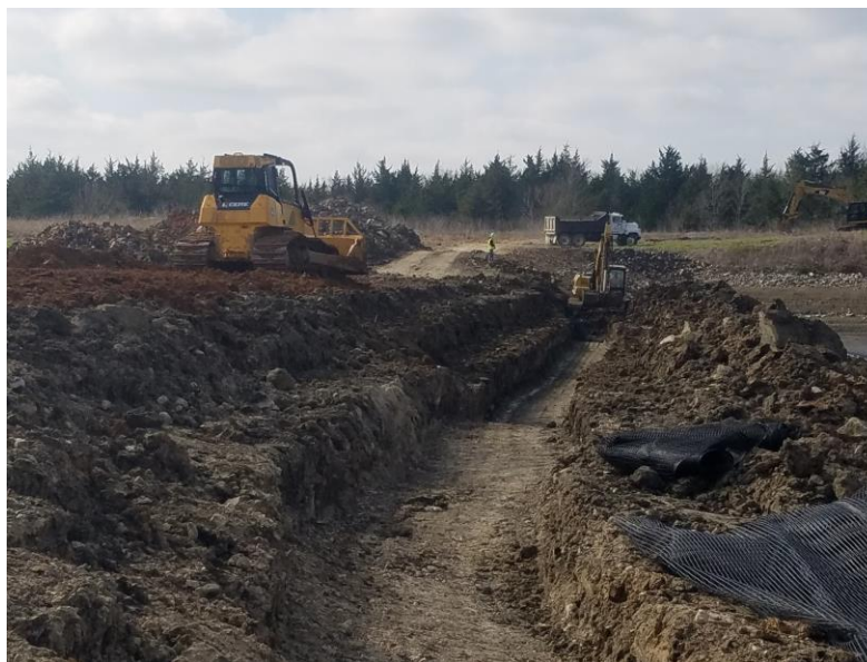
FIGURE 6: EXCAVATING THE SOIL AROUND THE SLIPPAGE CRACK
