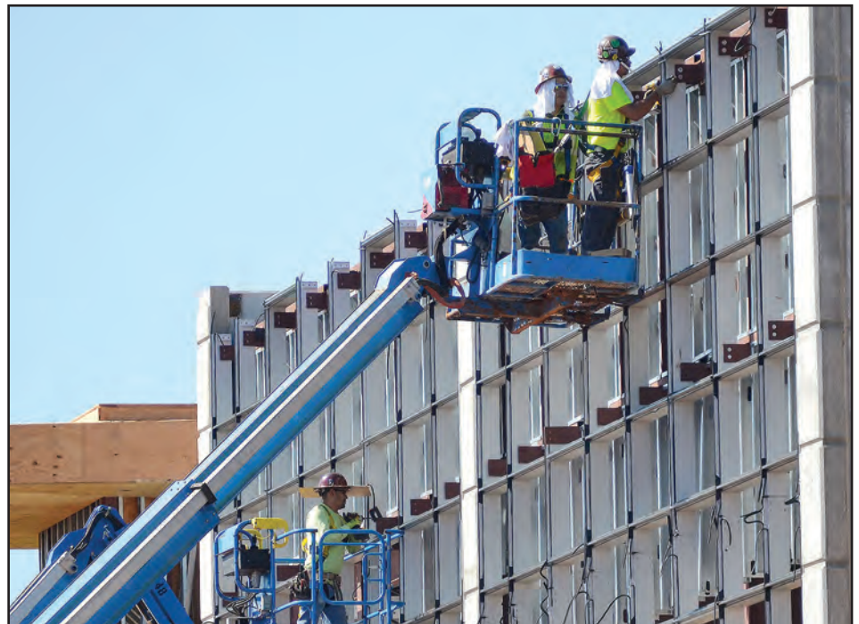
During 2018, construction continued on the new Moore Office facility, which should be ready for occupancy in April 2019. Weather was a factor when preparing and paving the parking lot, which caused delays both inside with deliveries and outside construction.
