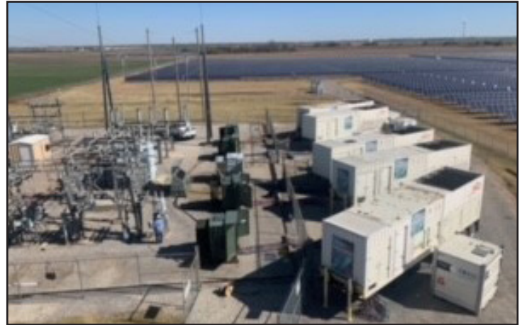
Distributed generation (DG) units have been placed at the Tuttle Substation and are set to be energized around noon today. This step will help energize that site while transmission repairs continue.
