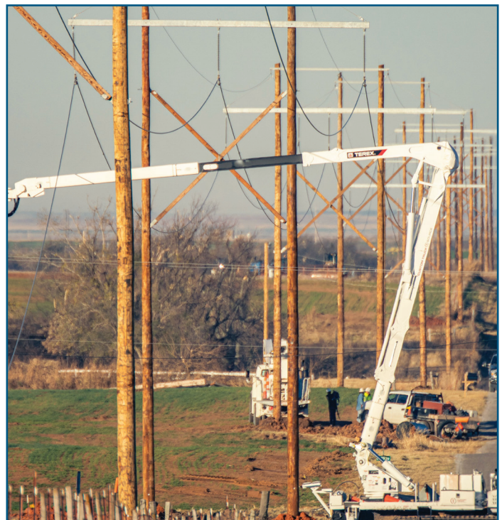
Newly constructed transmission lines are shown as conductor is restrung between the structures. Contract crews were hired to assist WFEC crews with restoration efforts following the October ice storm.
